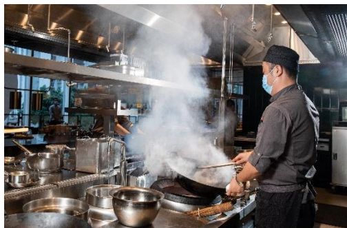
Kitchen Exhaust Fan at FEAST
